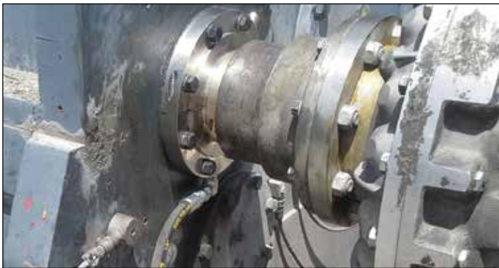
An external drain was designed to accommodate the operational flood in the Sag Mill Gearbox bearing housing.
